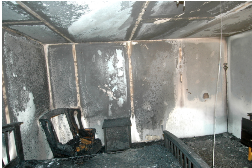
Fig. 1 - Cell 1 – This fire was extinguished at flashover. The origin is at the left side of this photograph. The patterns on the wall and ceiling above the nightstand were created late in the fire when turbulence moved the fuel gas from the oxygen deficient area in the left corner to where it could burn. The white wall area at the lower right is unburned.
