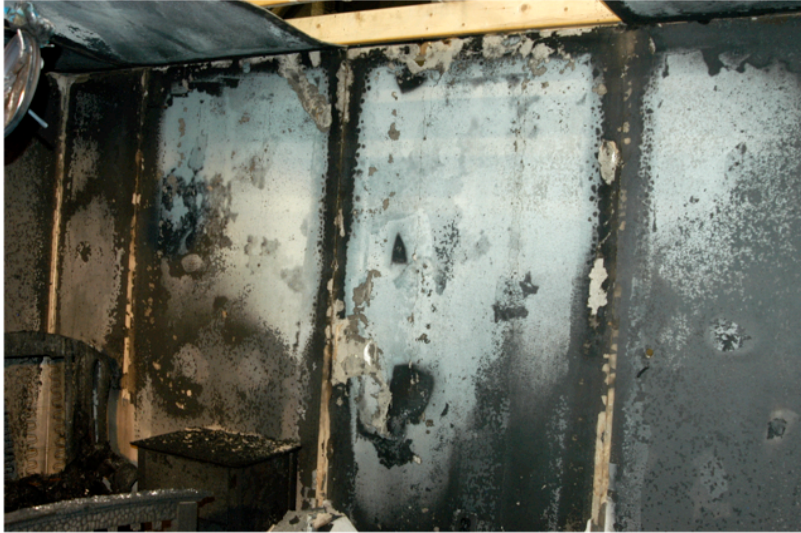
Fig. 2 - Cell 2 – This fire also set to the left of this photograph burned two minutes post-flashover. This pattern could be interpreted as a classic “V” pattern, pointing downward towards the origin. It was generated wholly from fuel rich gases migrating from the left and burning from the top downward as they encountered fresh oxygen. It does not mark the origin.
