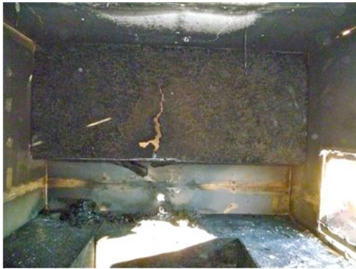
Figure 6 – View of area of origin. The pan of burning oil was on the lower cabinet
