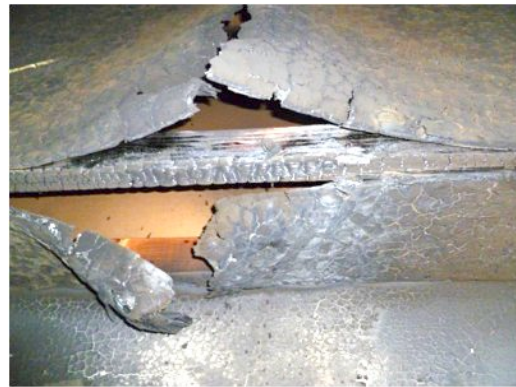
Figure 7 – Underside of cabinet directly above the origin
