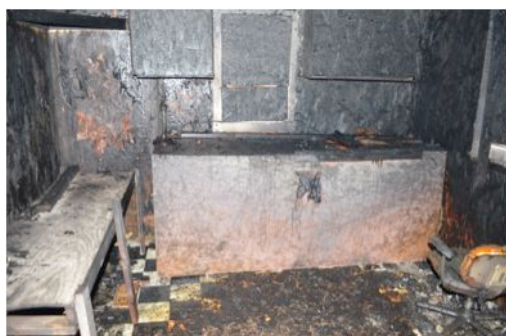
Figure 11 – Rear room. Origin at right side of lower cabinet. Top of the wooden table at the left is unburned.
