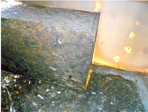
Figure 4 – Minor damage to wood cabinet and gypsum wall board in room of origin
