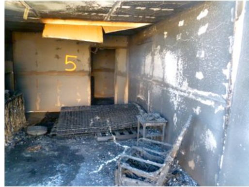
Figure 3 – Opposite end of large room showing areas with less damage. Room of origin is beyond distant doorway
