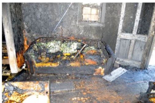
Figure 9 – Left side of front room. Open exterior door to the left. Room of origin is to the right
