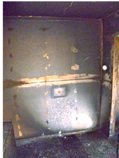
Figure 5 – Pattern on kitchen wall opposite origin. Door to larger room opens to the right
